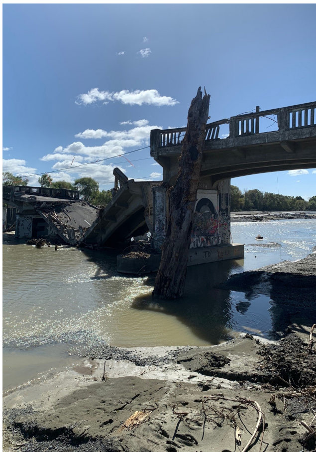
Redclyffe Bridge, Waiohiki, Hawke's Bay, extensively damaged by flooding during Cyclone Gabrielle in February 2023. Credit: University of Waikato
